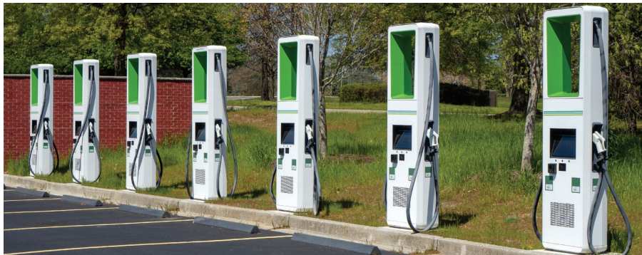
Figure 22.3 Charging stations are often underutilized.
